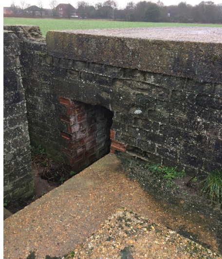
Figure 8 - View of the centre of the pill box with star and opening into enclosed room
